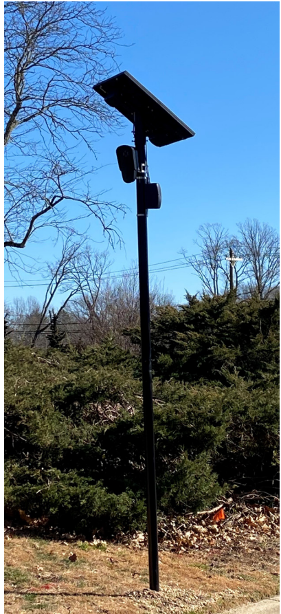
Solar powered ALPRs with LTE capability can easily be deployed anywhere with sufficient sunlight.
